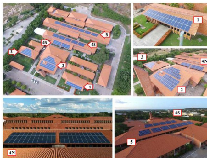
Figure 3 – Detailed view of the GCPVS installed at IFPI's Floriano Campus. Source: Morais et al. (2019).
