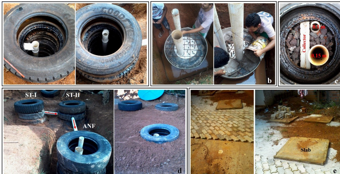
Figure 7 – Assembly and fixation of ST-I and ST-II (A); arrangement of pipes, construction of the concrete plate (false bottom) (B); filling of the AnF with gravel and installation of the treated sewage adhesive tube (C); drilling of the units and final arrangement (D); closure and system design (E).
