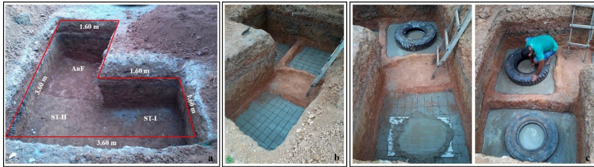
Figure 6 – Excavation of the trench for accommodating the TIRE-ATS (A); concrete piece at the bottom of the trenches (B); fixation of tires at the base of the units (C).
