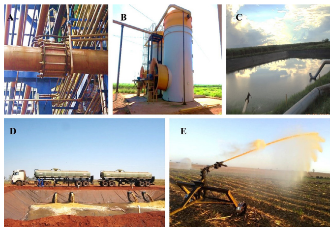
Figure 1 – (A) Automatic flow rate meter at the outlet of the distillation column, (B) Vinasse cooling towers, (C) Vinasse reservoir inside the industrial park, (D) Waterproofed reservoir in the agricultural area with unloading of vinasse transported by truck, and (E) Application of vinasse to the crop with a self-propelled irrigation system.
